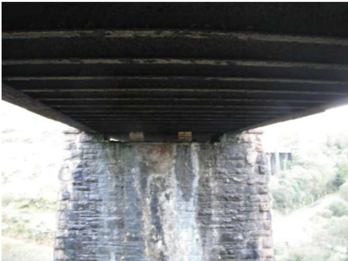
Figure 5 : Piers showing signs staining due to water percolating through expansion joints.
