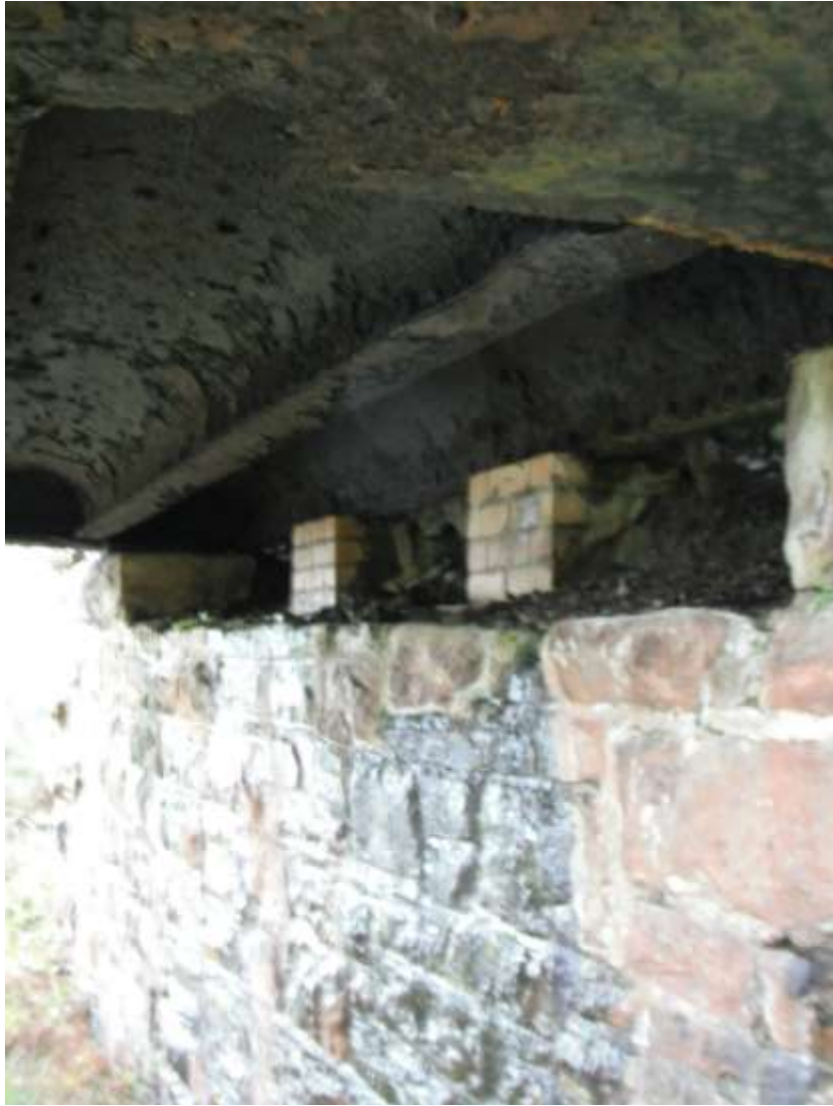
Figure 6 : Abutment - note the lack of bearings.
