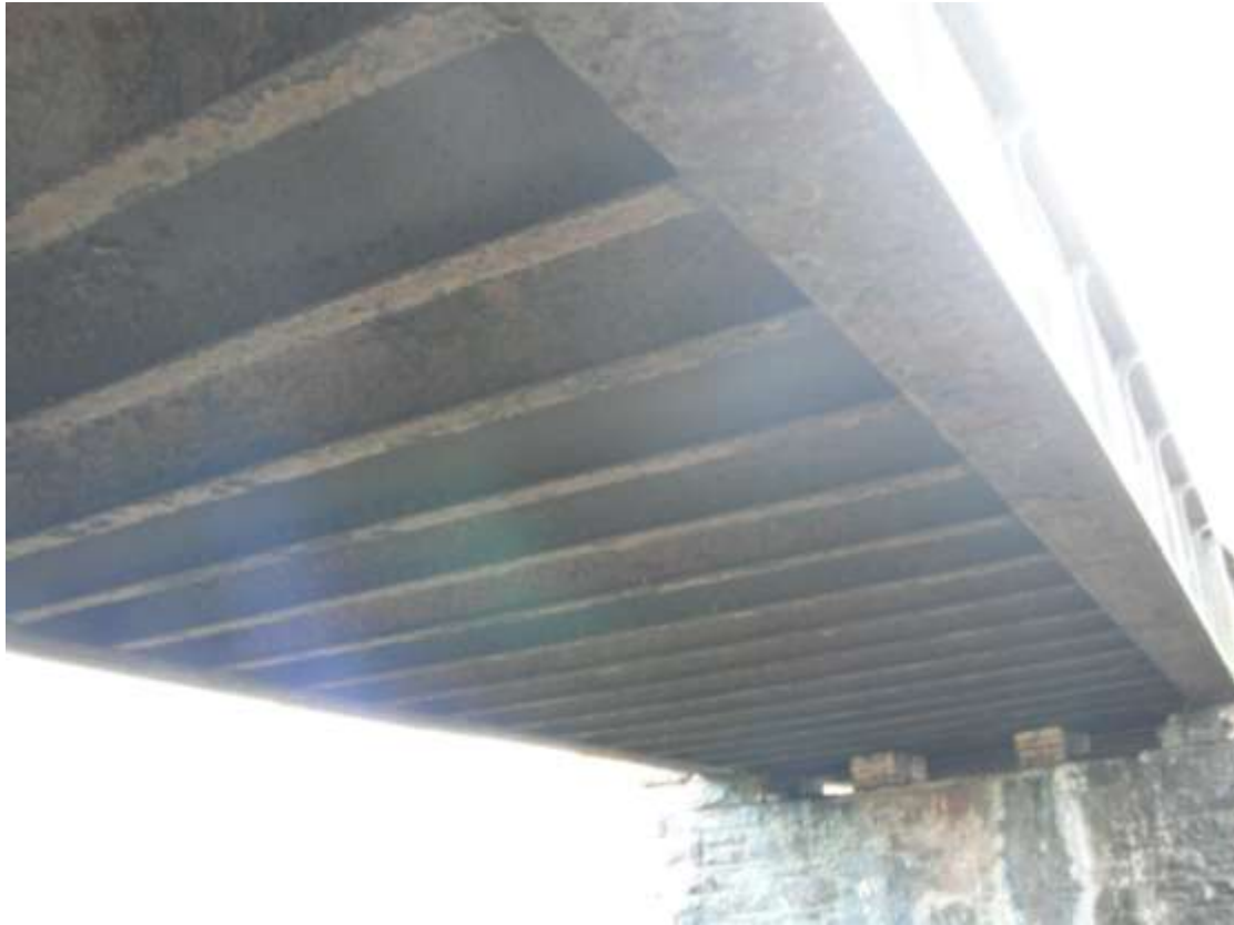
Figure 4 : Deck soffit showing minor corrosion to transverse beams.
