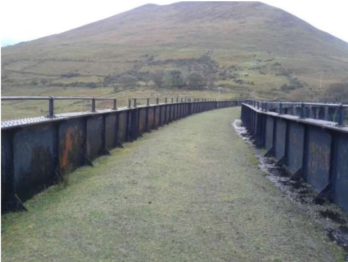
Figure 2 : General view along deck showing plate girders, build-up of stone/soil material and CHS handrailing.
